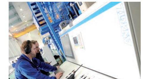
Complete plant automation
