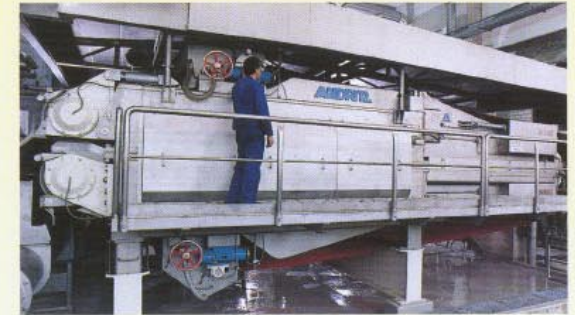
Twin-Wire Press in a HC-bleach plant
